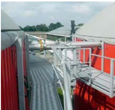
Installations de biogaz
